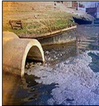
Sewage Spill May be Manhole Leak Threat to health & recreation
